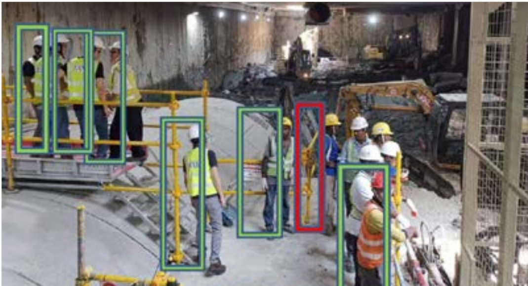
SAFETY RULE VIOLATION DETECTION
